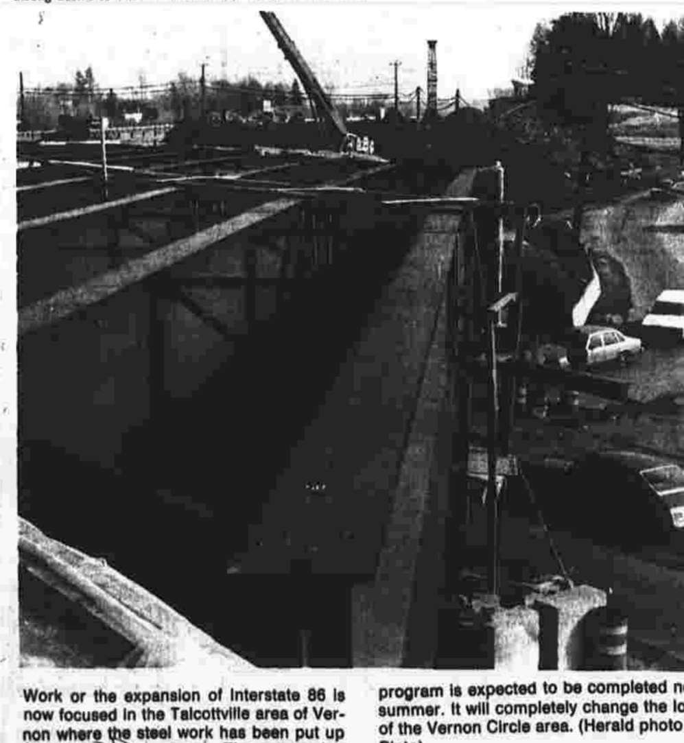
Work on the expansion of Interstate 86 is now focused in the Talcottville area of Vernon where the steel work has been put up for the new overpass. The expansion program is expected to be completed next summer. It will completely change the look of the Vernon Circle area. (Herald photo by Pinto)
